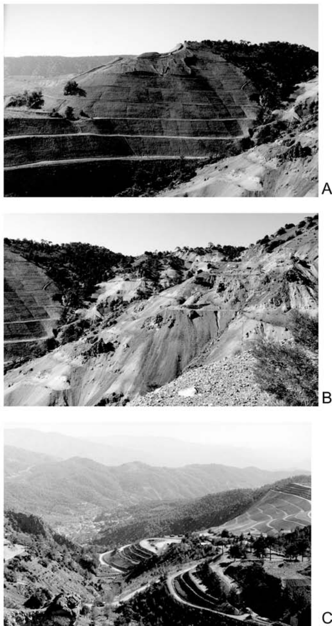
Figure 6. Remediation work in progress on the now-closed Cyprus chrysotile asbestos mine. A: Photograph of engineering work involving lowering the angle of repose of the talus slopes by the construction of an intervening series of benches between the slope sections. B: Photograph of to-be-stabilized talus slopes (right) and stabilized slopes and benches (left). C: Photograph of partially completed slope and bench reconstruction (right), as well as a view down the stream valley toward the town of Kato Amiantos (left center).
